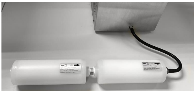
Zero filter installed
