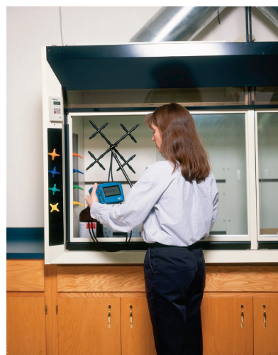
Figure 15. Face velocity is the primary method of evaluating fume hood performance after initial set-up.
