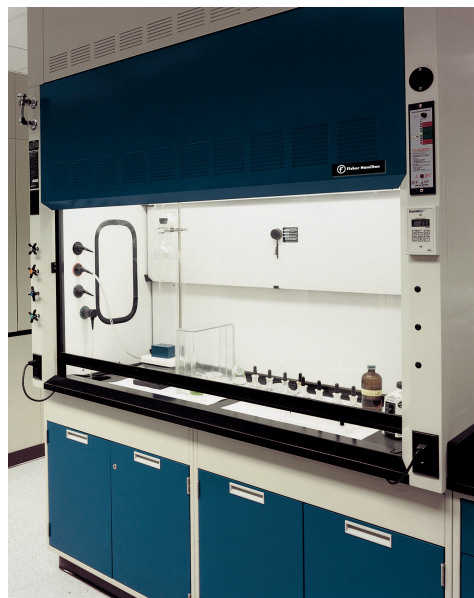
Figure 13. Benchtop fume hood. Photo courtesy of Fisher Hamilton LLC.
