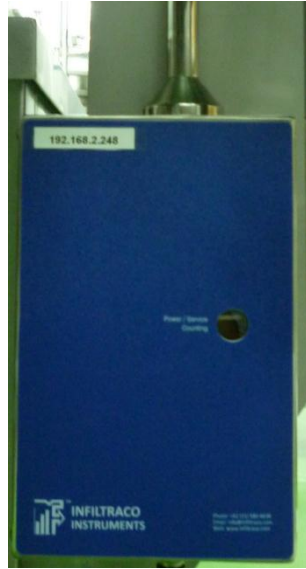
Figure 8. Remote particle counter installed in a Stainless Steel enclosure to prevent ingress of cleaning solutions.
