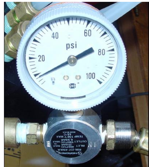
Figure 4: Pressure Gauge Showing the Inlet Pressure
